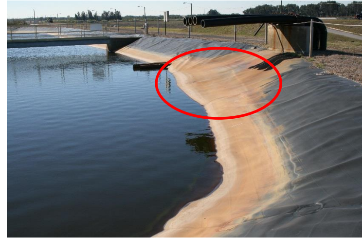
Economizer Ash Suction Pond (west side, looking south at irregular liner surface)
