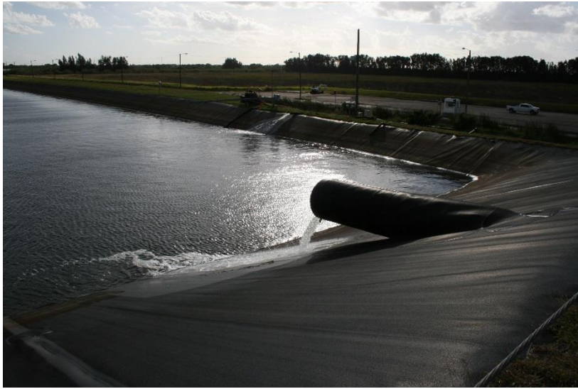
South Economizer Ash Pond (south side, looking southwest at bulge below central pipe discharging into the Long Term Fly Ash Pond)
