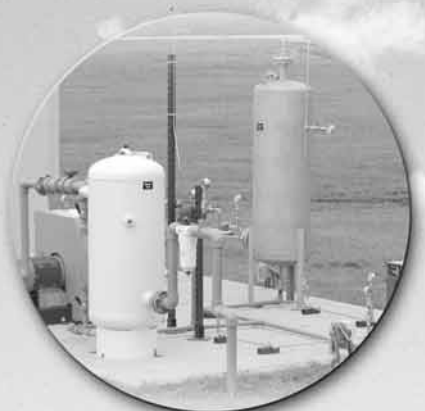
Methane gas produced by buried waste in Hillsborough County disposal sites is used to generate electricity.
