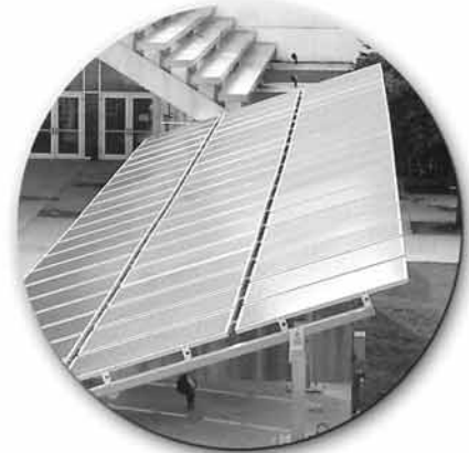
A solar panel array Tampa Electric installed at the Museum of Science and Industry produces clean electricity.
