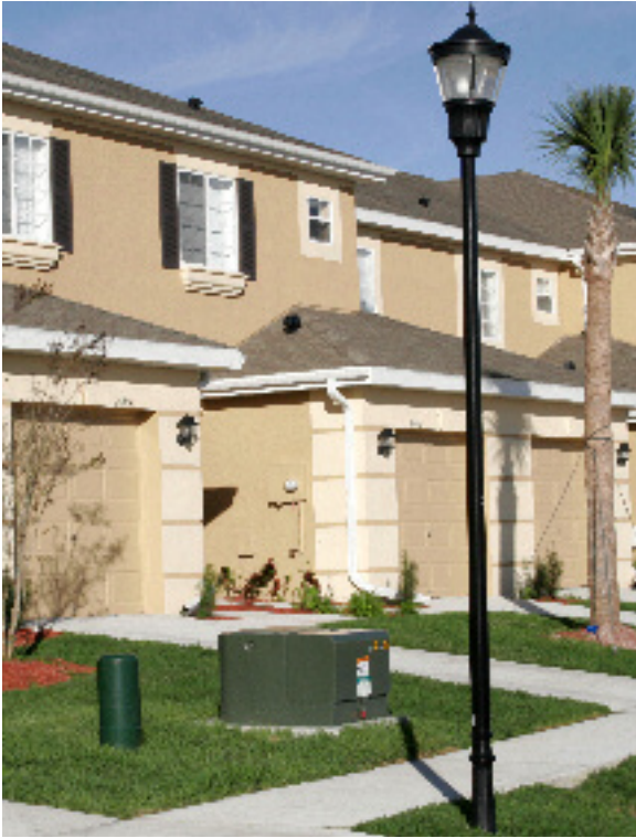
Underground electric service to a residential building.
