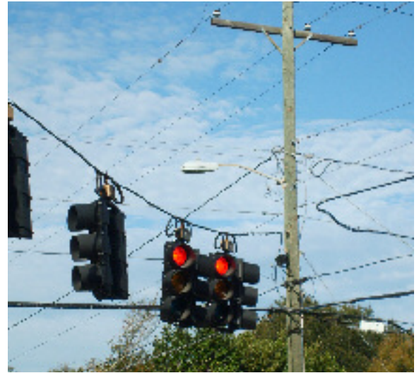
Overhead poles often support third party facilities such as traffic signals.
