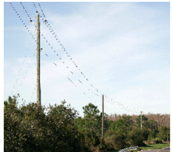
Overhead system without third party attachments on the electric poles.
