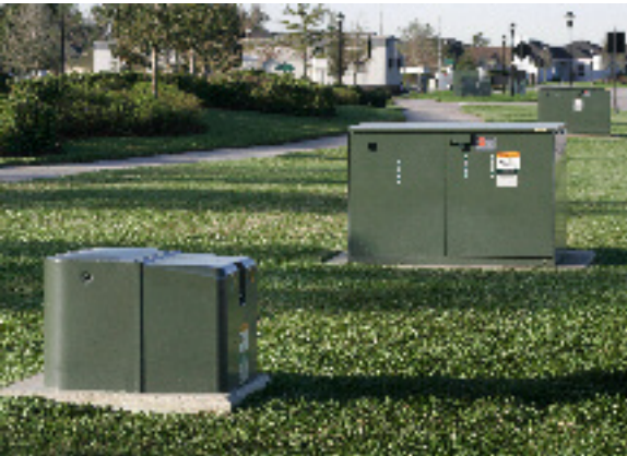
Easements are required for underground electric transformers and switches.
