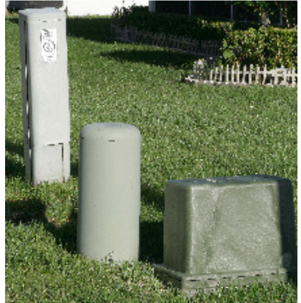
Underground system junction boxes for electric, communications and TV.
