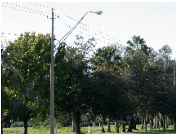
Overhead concrete poles.
