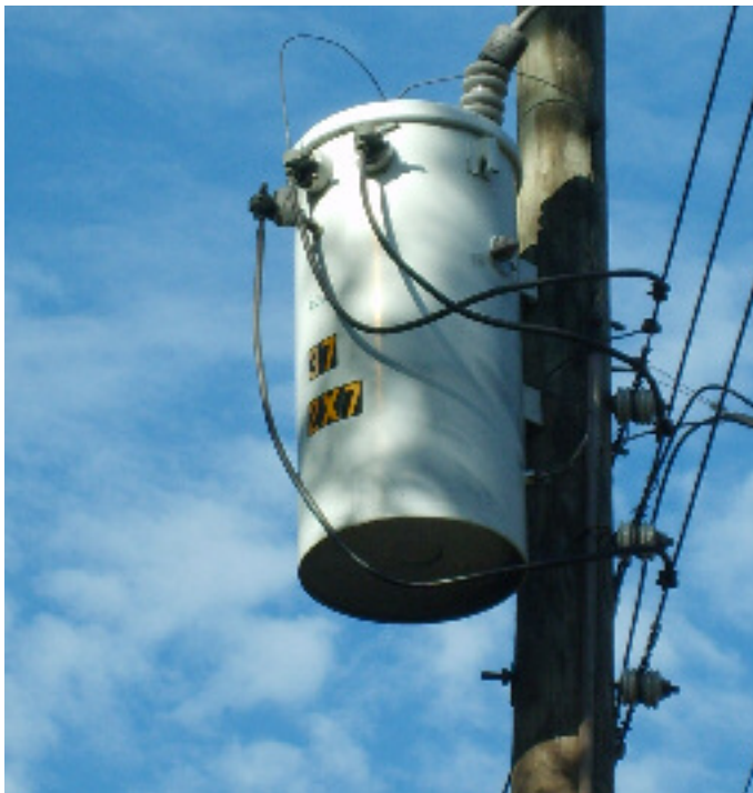
Overhead system single-phase transformer.
