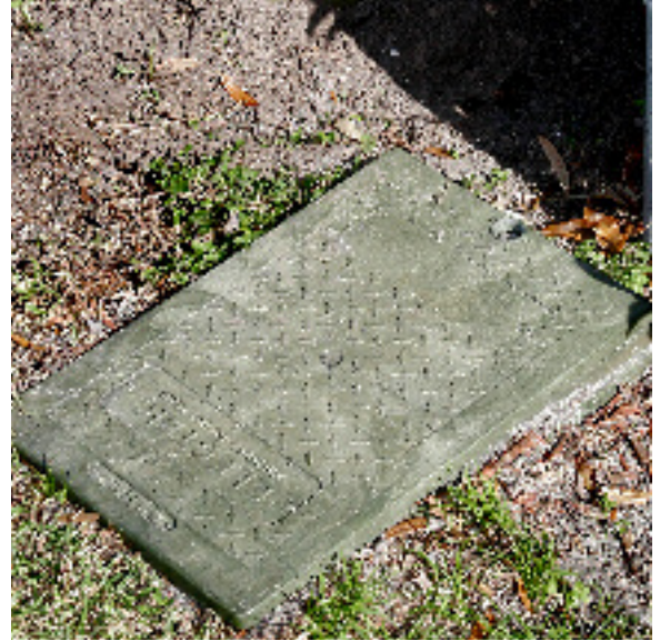
Underground service handhole from an overhead pole.
