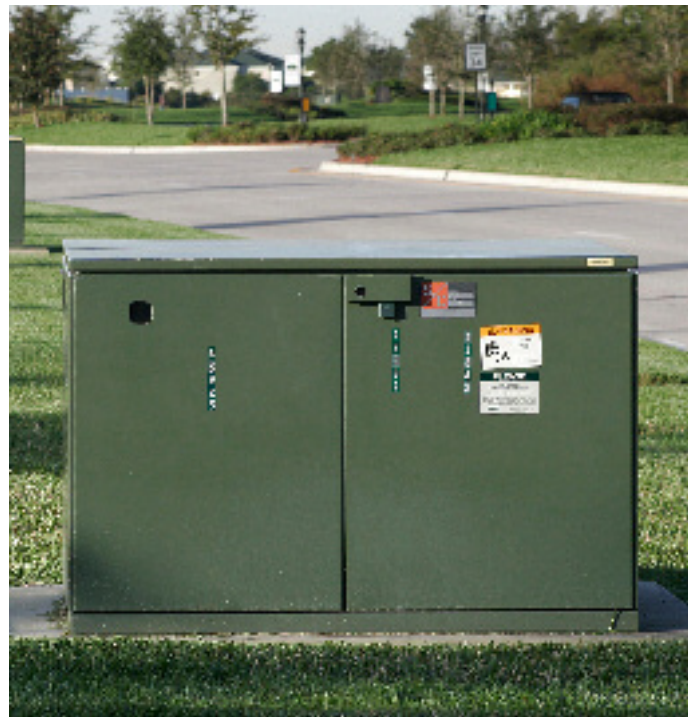
Underground system pad-mounted switchgear.
