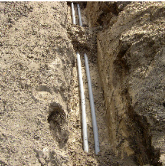
Underground electrical conduits in trench.
