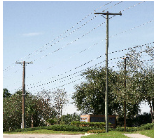
Overhead system communications cables supported from electric utility poles.
