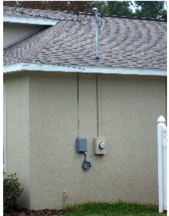
Overhead system service entrance.
