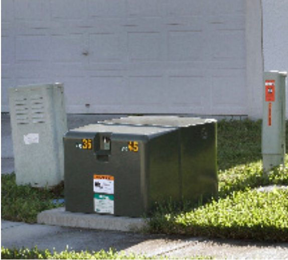
Underground system pad-mounted transformer and junction boxes for communications and TV.
