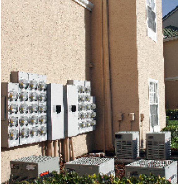
Underground electric service entrance for a residential apartment building.
