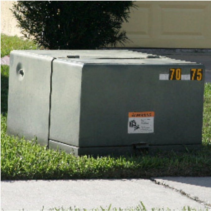
Underground system single phase pad-mounted transformer.
