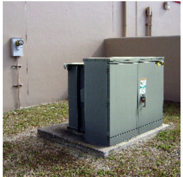
Underground system three-phase pad-mounted transformer.
