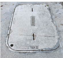
Pull Box or Splice Box
